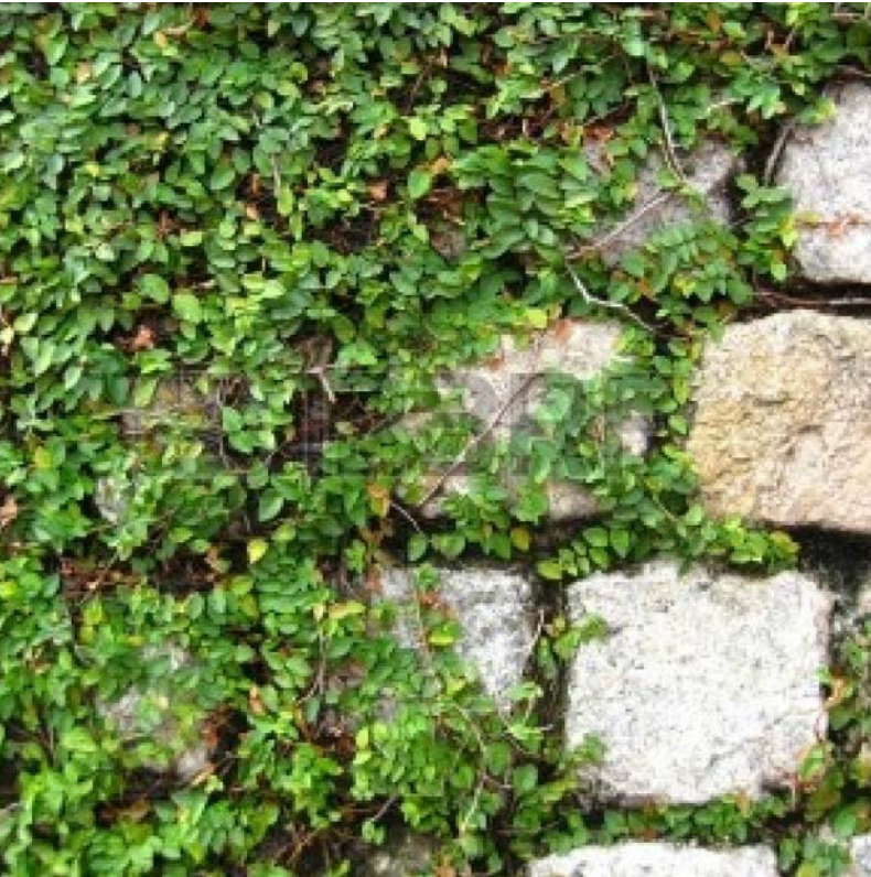
seeping out from cracks
